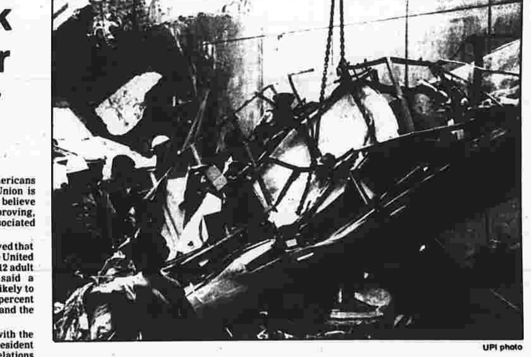
As civil defense searchers burrow into the mounds of the collapsed New World Hotel in Singapore, other workers cart away debris Sunday.
